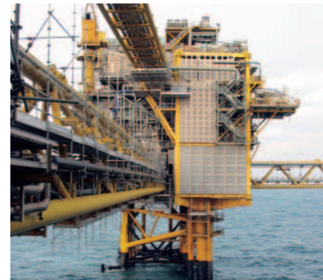
A caisson supported module extends the capacity of fully equipped platforms, Tyra Field.
