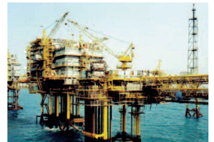
Additional external conductors installed on old platform, the Tyra Field.
